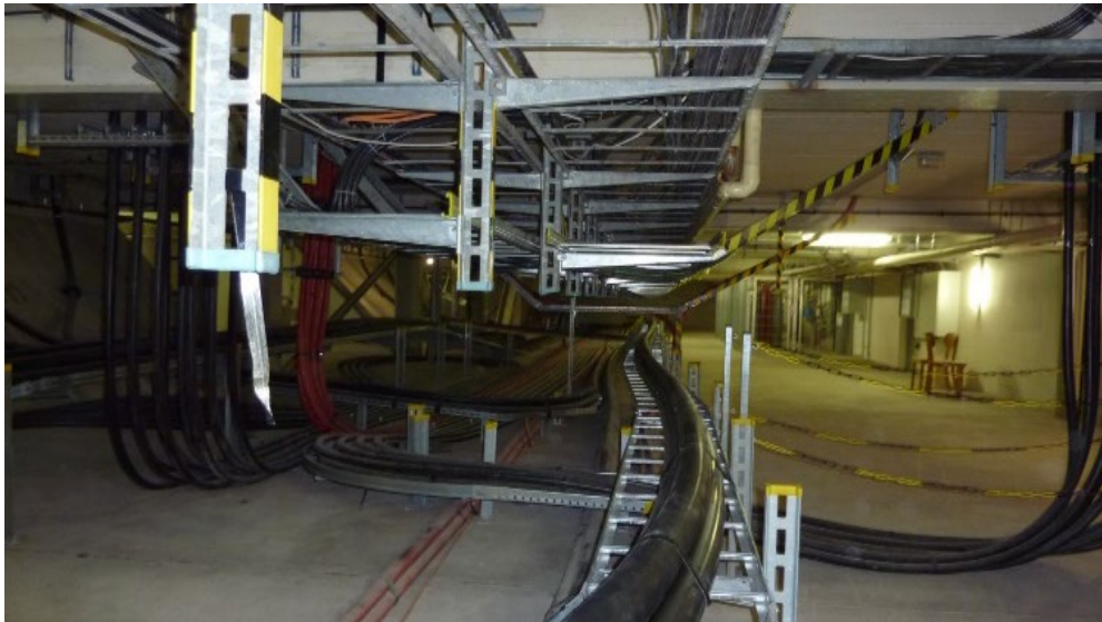
Trefoil configuration in the substation
