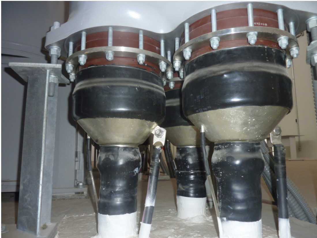
GIS termination showing the three phases
